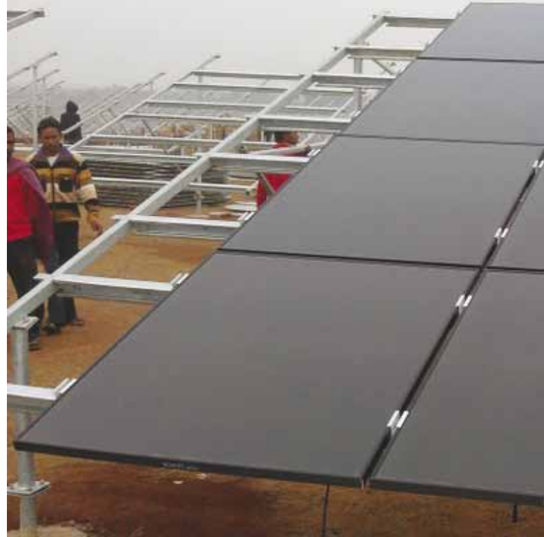
6 MW Premier Solar, Deoghar, Jharkand
